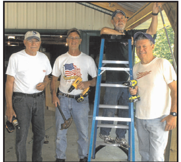
Volunteers Jack Kloss, Tom Braunreiter, Gene Golsschmidt and Larry Sommer doing the electrical in the new pavilion.
